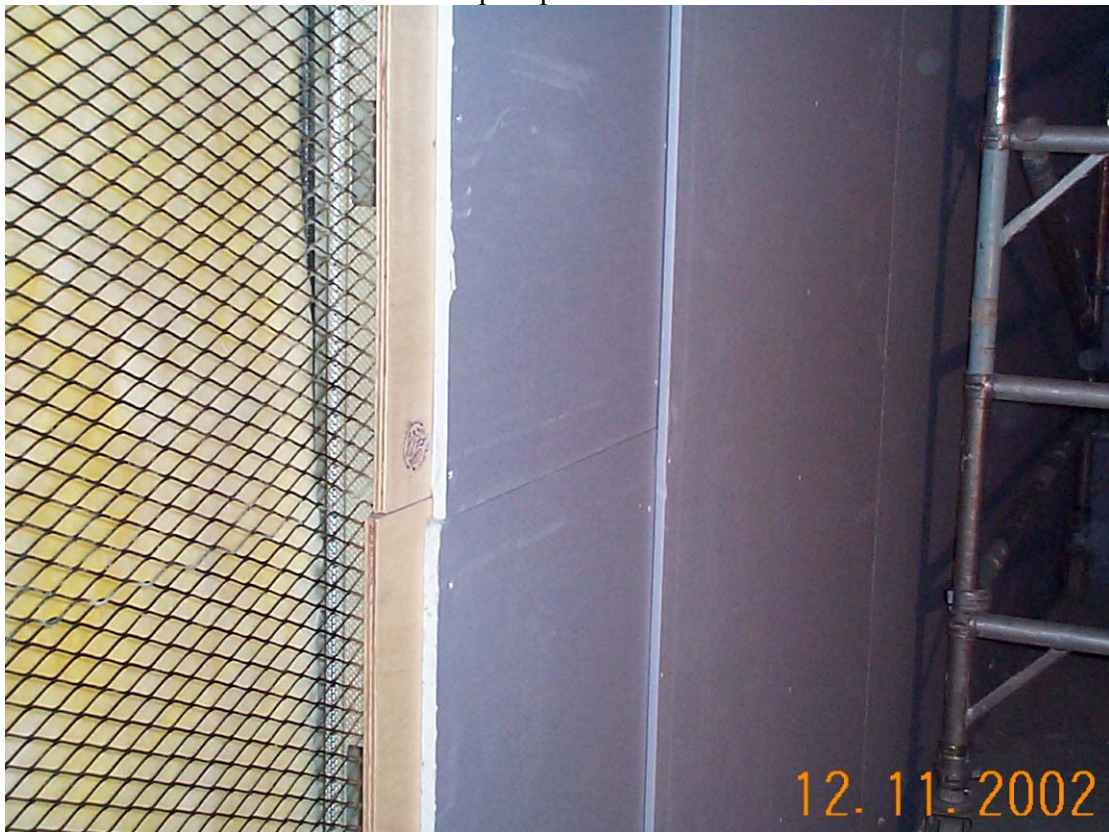
Figures above & below show the Audio wall detail, Isowool acoustic insulation, Expamet security lath, WPB plywood and two layers of BG soundbloc. A fire rated deflection head was also installed as per specification.
